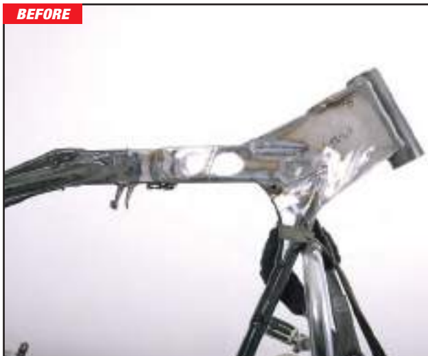
The HHI neck rake kit has been installed and Project 04' Road King is now ready for the new front end.
